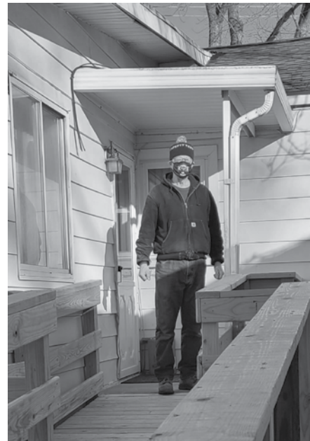
Bill Helwig posing on the newly installed deck he volunteered so generously to build.
